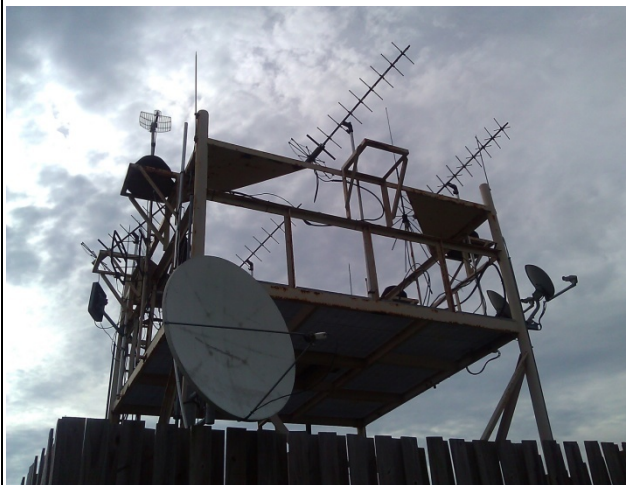
Figure 2: Special Operations Command South Antenna Cluster
