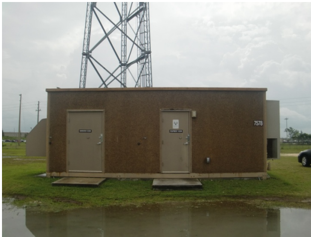
Figure 7: Motorola Quantar Repeater Control Building
