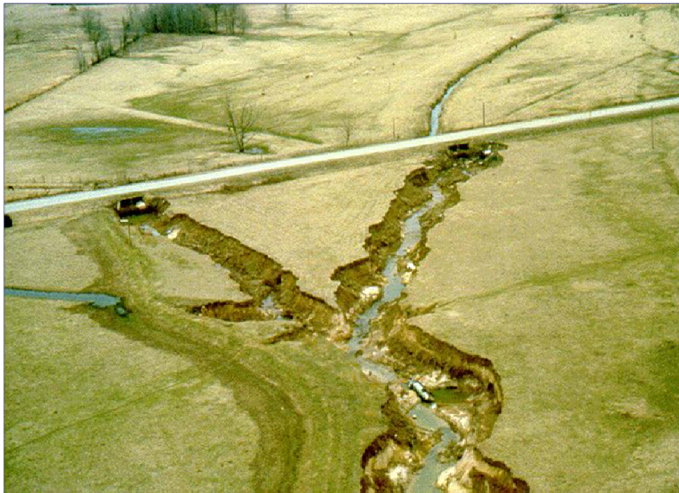
Figure 3. Channel degradation halted by two culverts on Crowder Creek. The culverts are acting as temporary grade control structures.
