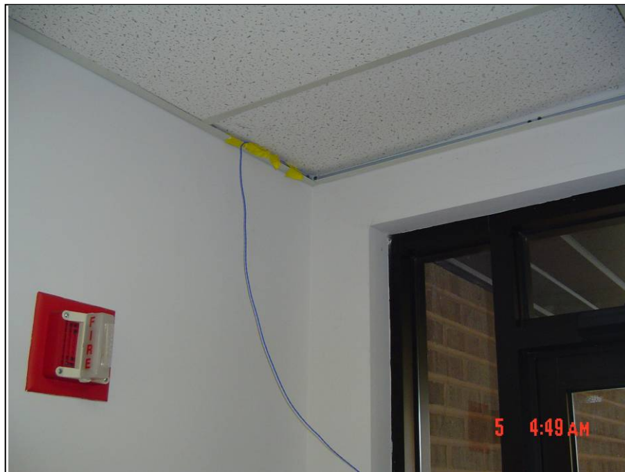
Figure 3-29. APG Building 2006: Horizontal Uniaxial Accelerometer Array for Location 5, E of S Front Door Entrance (to right is S)
