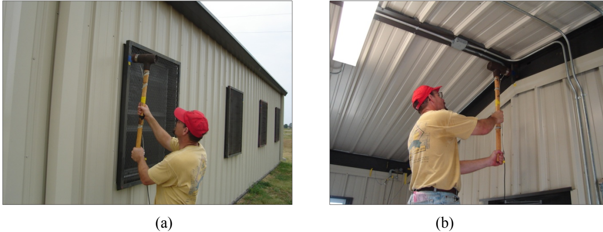
Figure 3-62. Fort Sill, Hammer Testing at (a) Exterior and (b) Interior of Building 6429.
