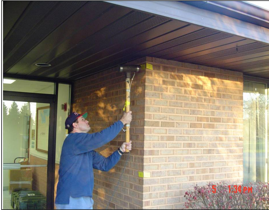
Figure 3-36. APG Building 2006: Close Up View of Front Door Entrance (to right is S) In this view the hammer has impacted the brick veneer wall near the top (near ceiling height) in the east direction (Location L in Figure 3-32)
