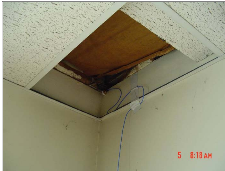
Figure 3-43. APG Building 4031: Interior View of the Transducer Mounted Above the Ceiling in the Southwest Corner
