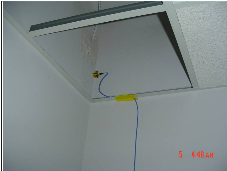
Figure 3-26. APG Building 2006: Horizontal Biaxial Accelerometer for Location 2, NE Corner (to right is S)
