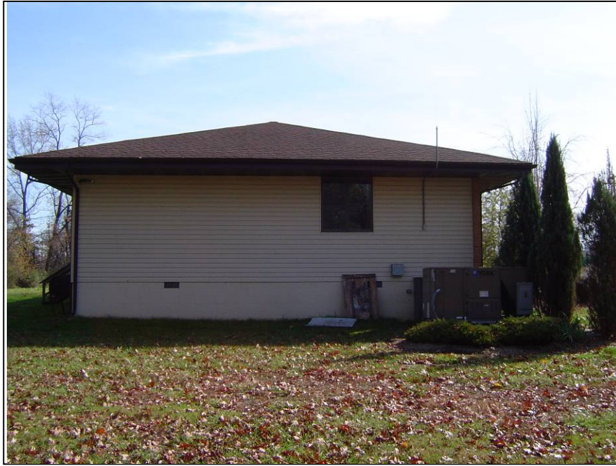
Figure 3-21. APG Building 2006: Side View of the West Exterior (to the right is S)
