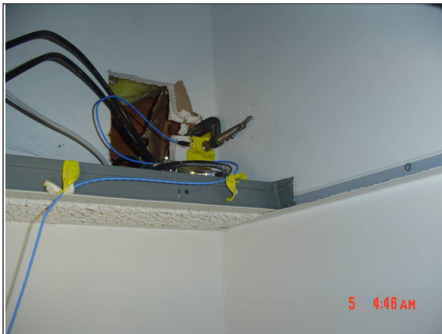
Figure 3-25. APG Building 2006: Horizontal Biaxial Accelerometer at Location 1; Interior SE Corner Above the Drop Panels of the Ceiling (to right is S)
