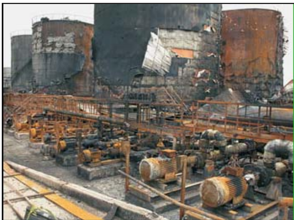
Figure 3-6: Destroyed Tanks and Pipelines at Novi Sad Oil Refinery
