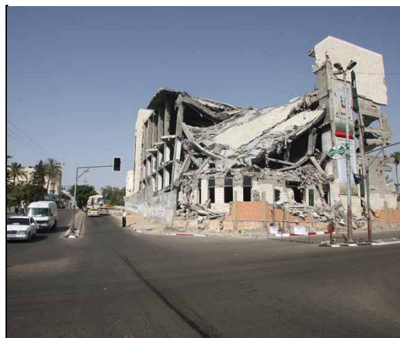
Figure 3-17: Partially Demolished Building in Gaza City
