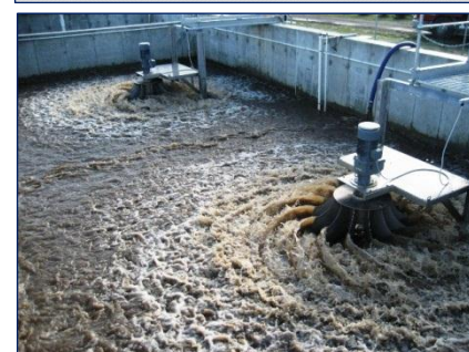
Figure 10. Sequencing Batch Reactor
