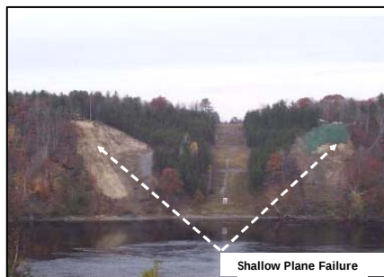
Figure 34. Shallow plane failure.
