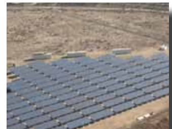
DoD IG reviewed DoN photovoltaic Recovery Act projects.
