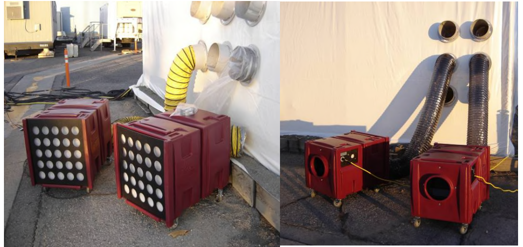
HEPA negative air filters being used to reduce building VHP levels
