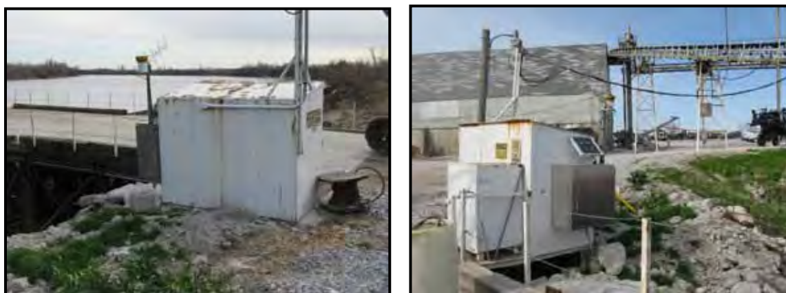
Figure 10.35.2 – Brunswick Terminal DCP. DCP gage house attached to electrical shack at main dock (left). Gage house looking toward terminal storage building (right).
