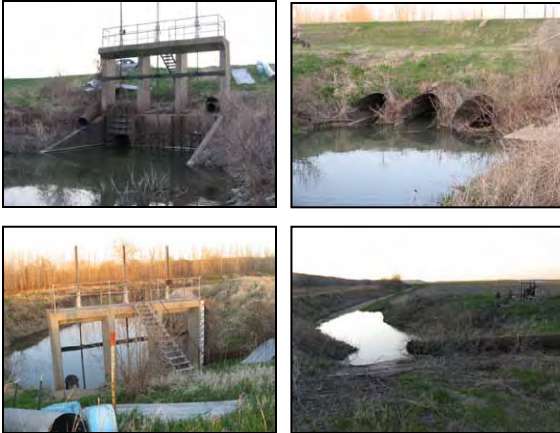
Figure 10.25.2 – R-500 site. Main outfall gate structure with screw-gated outlets (top left). Three 60-in. CMPs through main levee (top right). Main outfall gate structure and outlet ditch to river (bottom left). Inlet ditch of main outfall and fields (bottom right).
