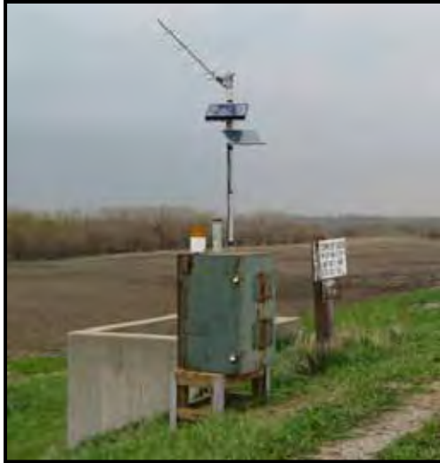
Figure 10.30.3 – L-408 DCP gage. DCP monitors both LS and RS water surface elevations.
