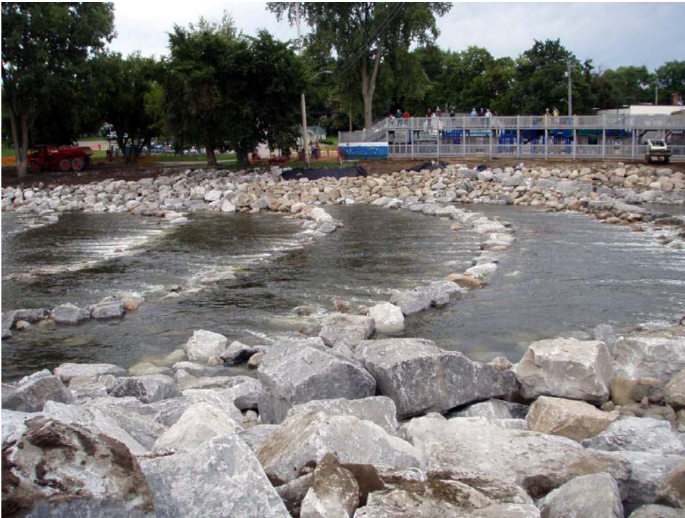
Figure 7: Typical rock ramp fish passage. Photo taken during construction, during low-flow period (August 2009). Site located in Chesaning, Michigan.
