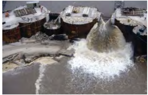
Flooding of second stage cofferdam, 9 October 1986
