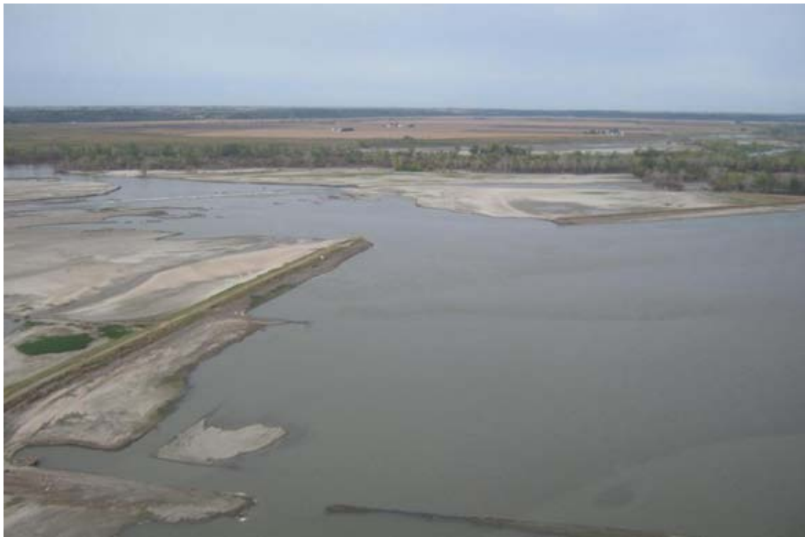
Figure 109. Levee breach: Lower breach at L575
