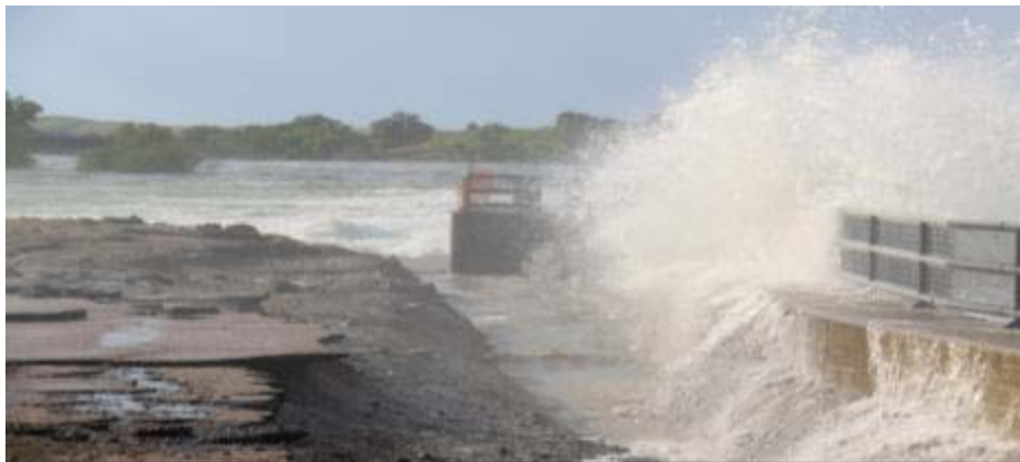
Figure 81. Dams damage/erosion: Oahe
