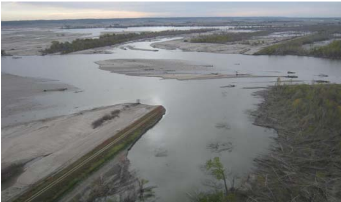
Figure 111. Levee breach: Upper breach at L550
