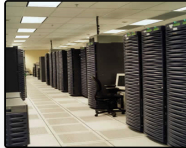
Hewlett Packard Cloud Computing Container
