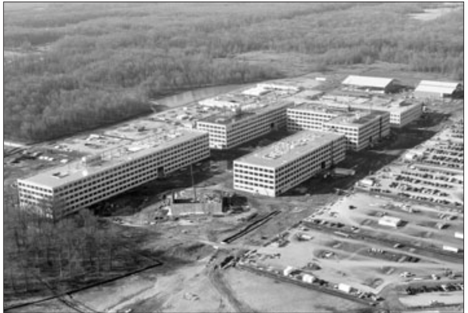
New facilities under construction at Aberdeen Proving Ground, Md., in 2008 for relocation of the Army's Team C4ISR from Fort Monmouth, N.J.
