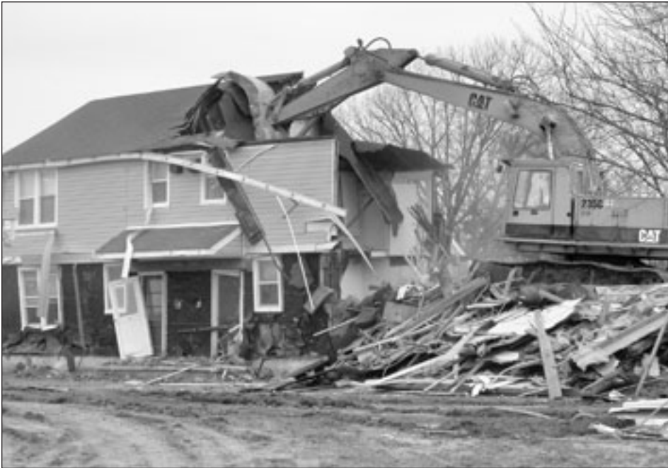
Military construction projects at McGuire Air Force Base in the 80s and 90s included both demolition (top) and renovation (bottom) of enlisted personnel housing
