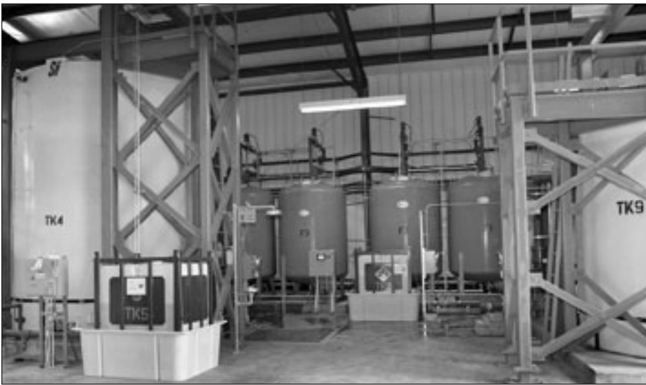
Groundwater treatment plant, Cosden Chemical Coatings Superfund Site
