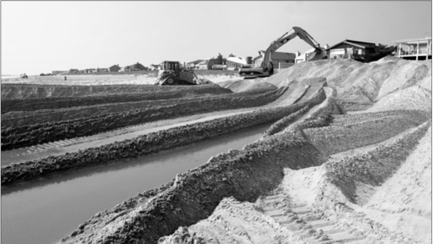
Initial nourishment at Fenwick Island, southernmost of three storm risk reduction projects covering Delaware's Atlantic Coast
