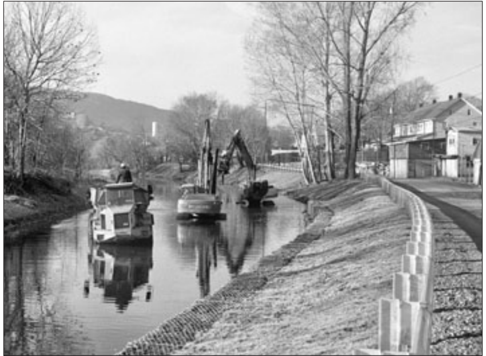
The Aquashicola Creek Flood Control Project in Palmerton, Pa., during construction (top) and after completion (bottom)
