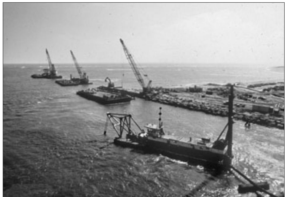
The plan for Barnegat Inlet involved construction of an entirely new south jetty backfilled with sand dredged from the inlet
