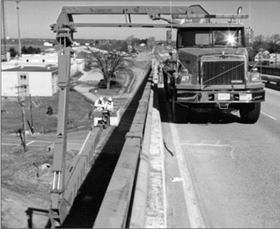
The Chesapeake City Project Office has specially designed truck-mounted equipment for below-deck bridge inspections and maintenance
