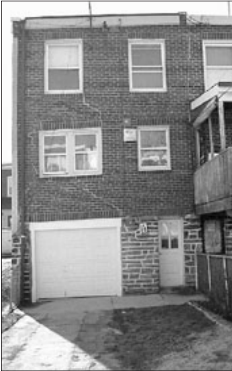
Visible settlement cracks characterized “sinking homes” such as this one in Philadelphia’s Wissinoming section
