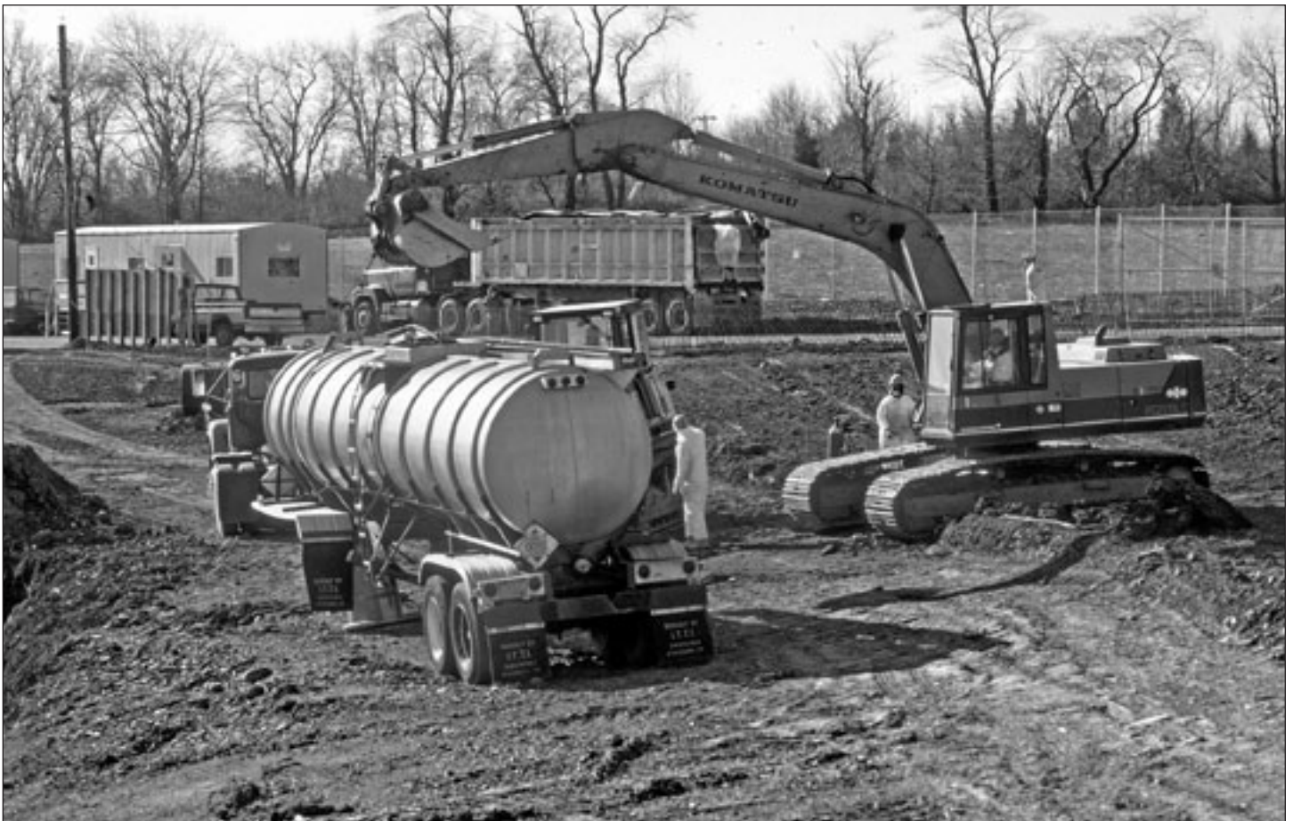
The Krysovaty Farm Site, the first Superfund cleanup completed by the Philadelphia District for EPA Region 2
