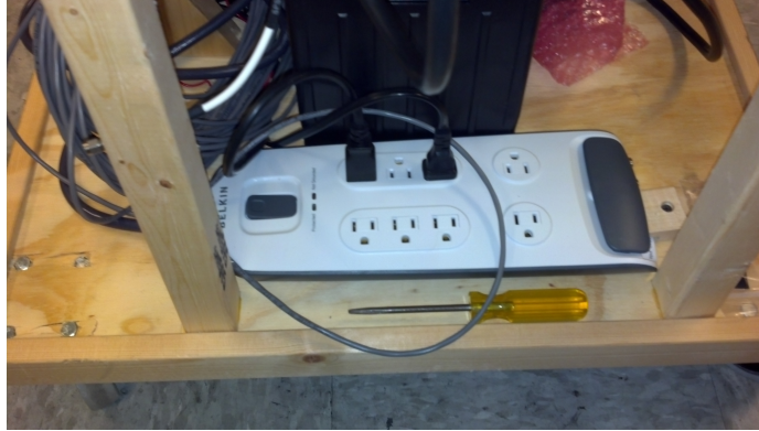
Figure C.2: Power strip for AFIT RNR
