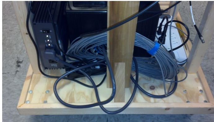
Figure C.1: Power strip plugged into AC/DC power inverter
