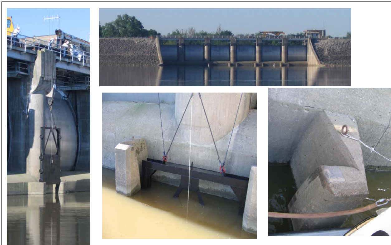
Figure 4-35. Steel service gate with binding issues.
