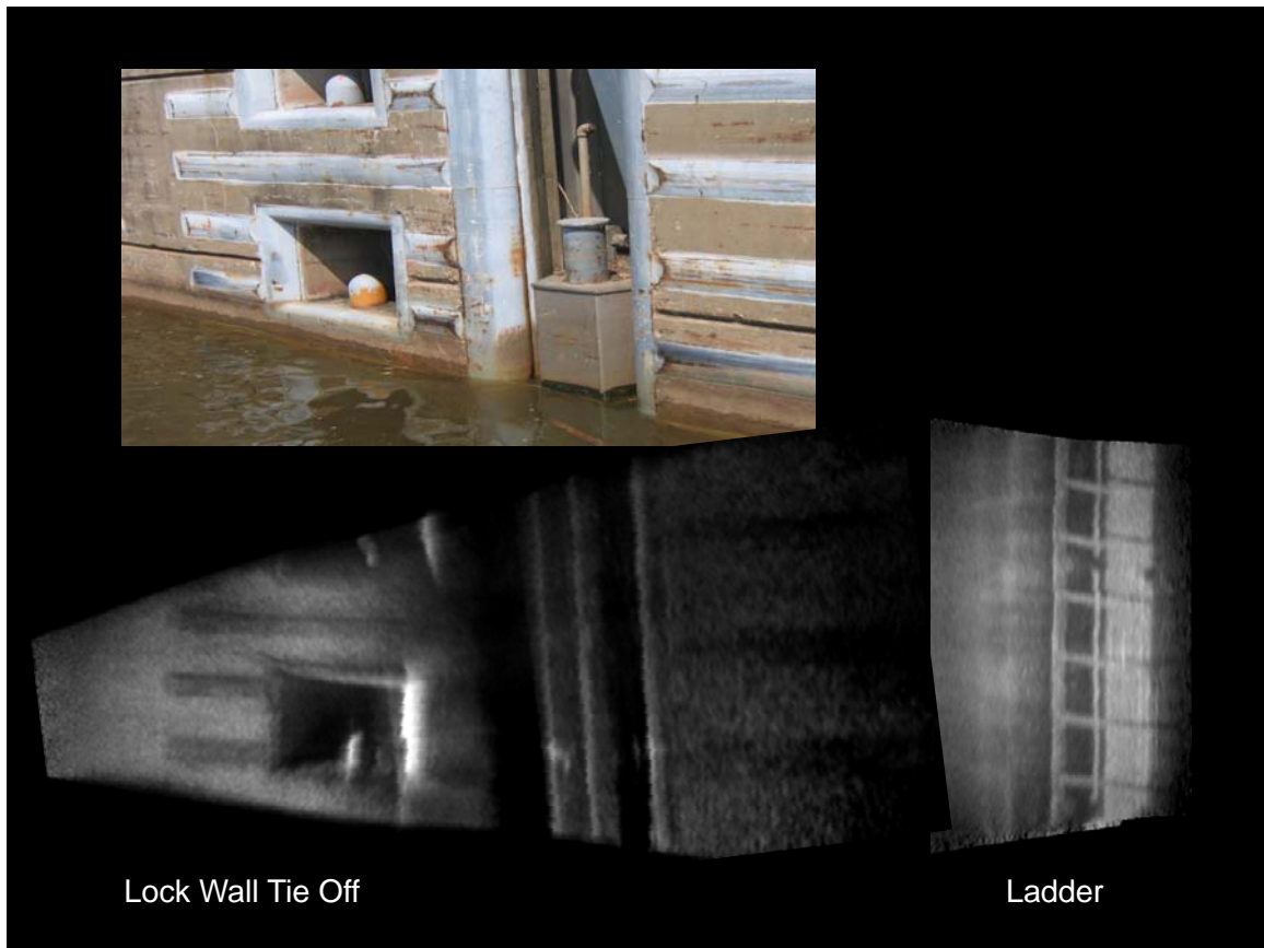
Figure 4-29. Acoustic camera mosaics of underwater lock components and a corresponding visible image.
