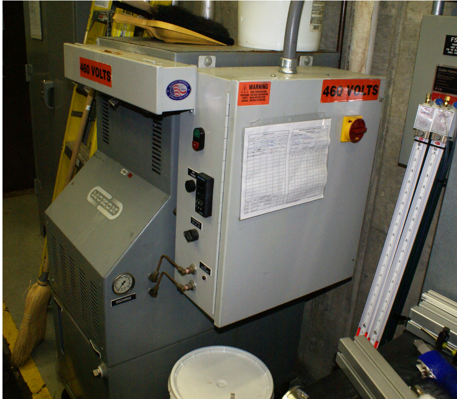
Figure 3.8: Oil Cooling System
