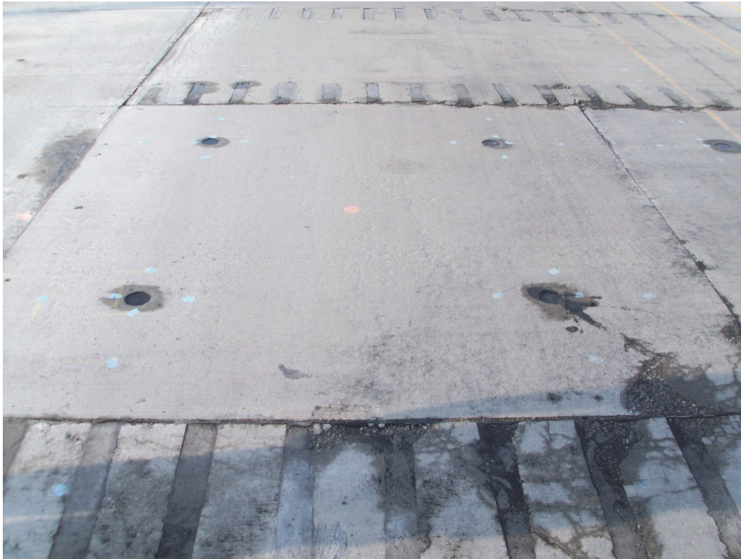
Figure 48. Repair 2-Panel 2 at failure condition.
