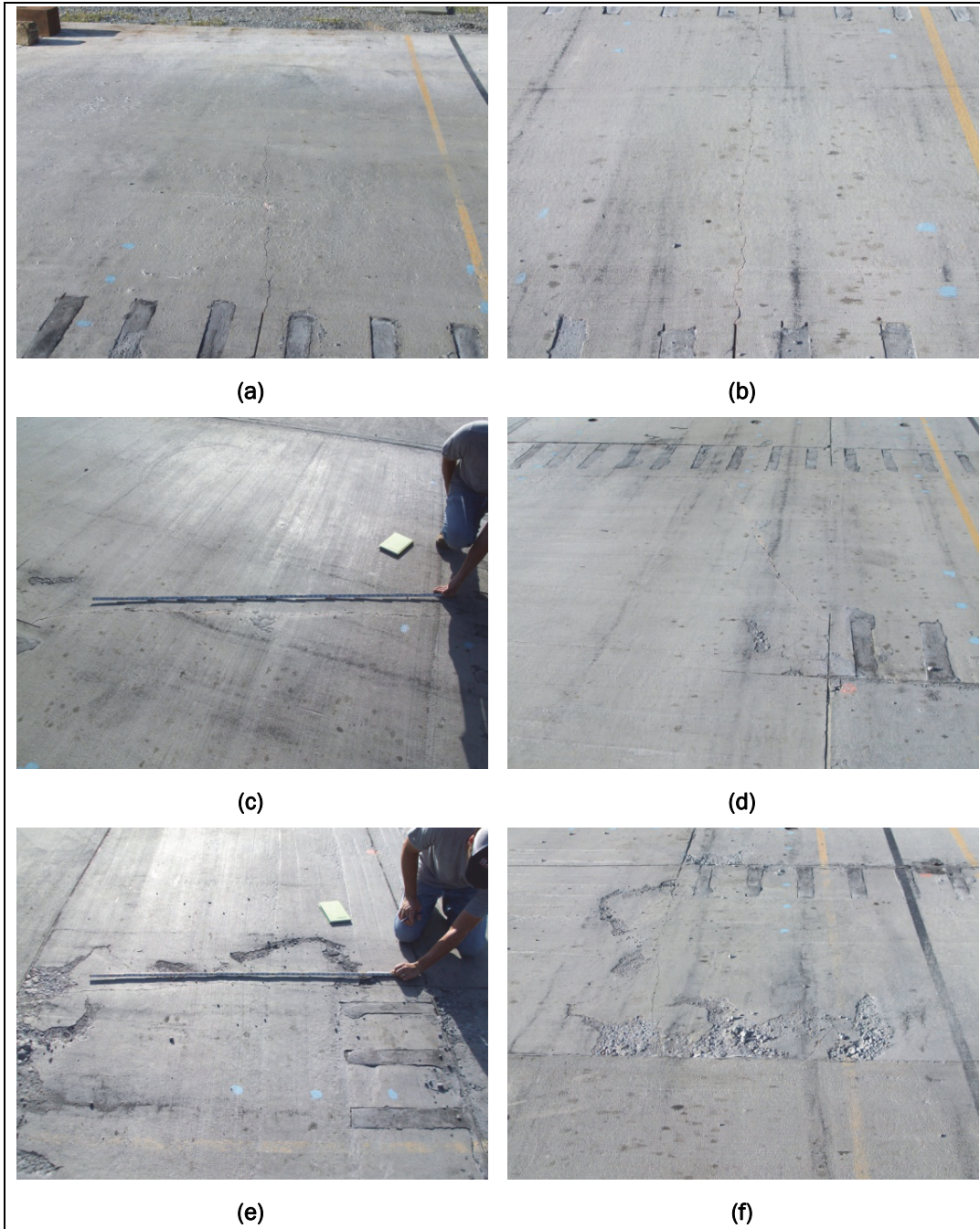
Figure 13. Parent slab distresses after 2,800 passes: (a) longitudinal crack in parent slab south of Repair 2 extending from saw undercut; (b) longitudinal crack in parent slab between Repairs 2 and 3 extending from saw undercut; (c) diagonal crack in parent slab extending from NE edge of Repair 1 extending from saw undercut; (d) diagonal crack in parent slab from SE edge of Repair 1 to Repair 2 extending from saw undercut and spalling and cracking between saw overcuts on SE corner of Repair 1; (e-f) spalling and cracking in parent slab north of Repair 1 near construction cold joint.
