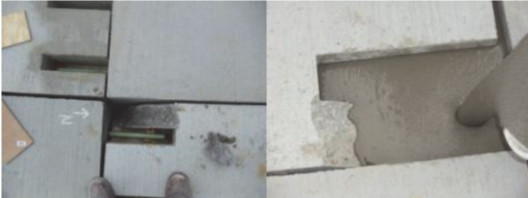
Figure 11. Damaged and repaired dowel bar receptacle on panel 4.
