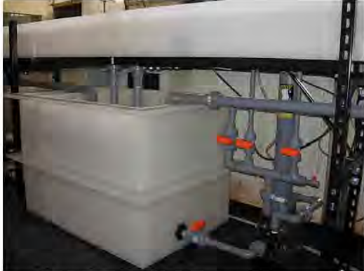
Figure 25 – Photograph of the electroplating sump tank showing the plumbing system. Solution is pumped from the side outlet near the bottom of the tank, through a fine particle filter column, and then fed up to the electroplating line cells above, which then drain back into the sump.
