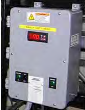
Figure 26 – Photograph of the temperature controller for the electroplating sump tank.
