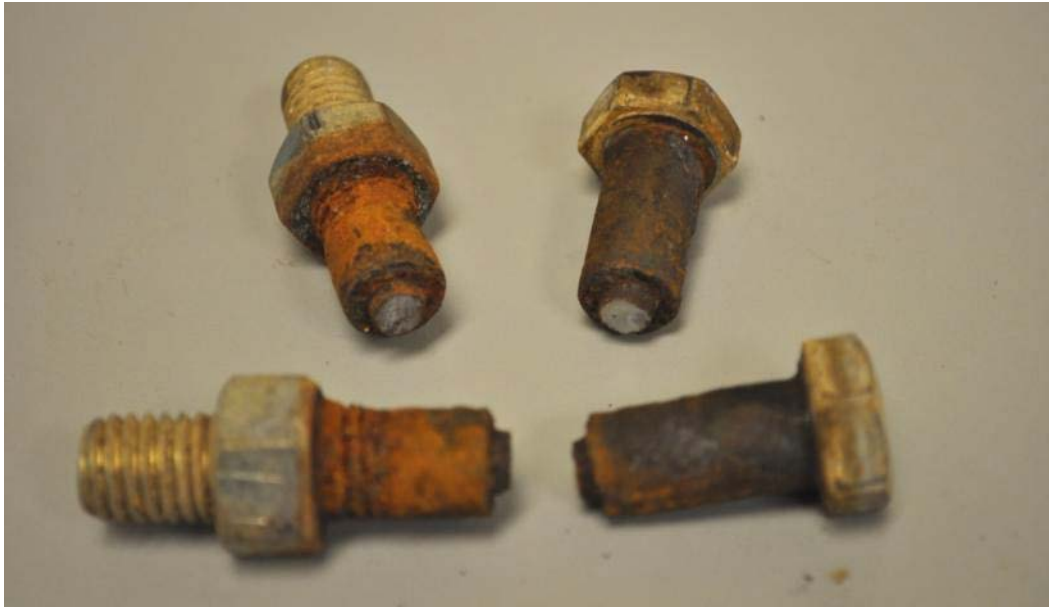
Figure 20. Corrosion on breakaway bolts 12 months after installation.
