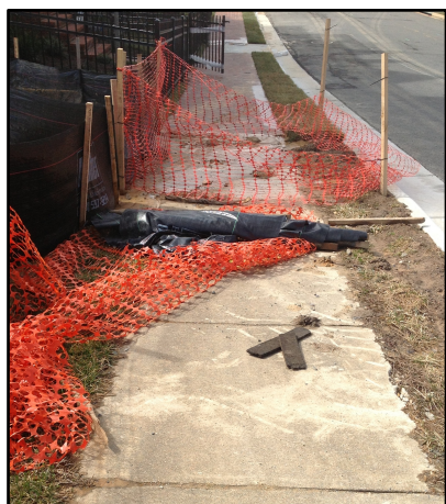
Figure 2. Construction debris and fencing temporarily blocking walkway
