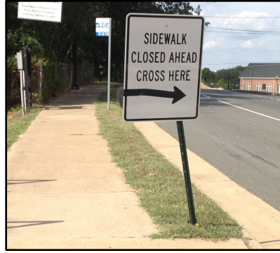
Figure 21. Signage added to facilitate crossing problem associated with detour
