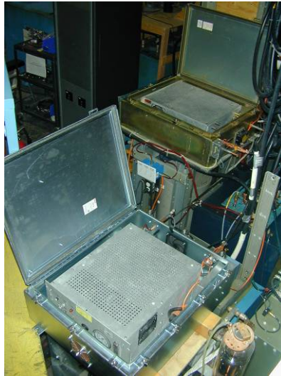
Figure 19. PI 40168 trigger amplifier in Hoffman enclosure
