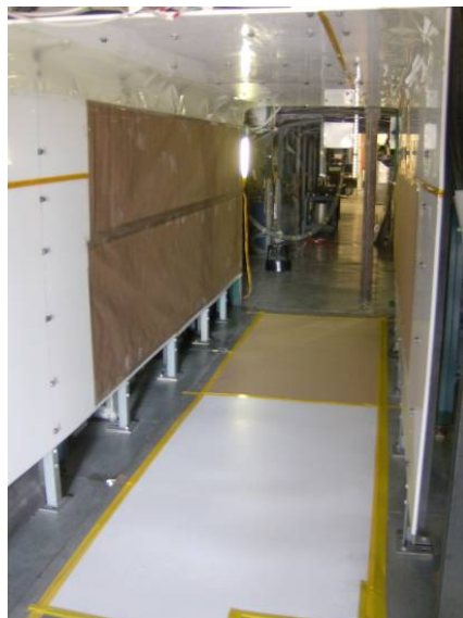
Figure 5. Floor, sides, and ceiling of the B-Arm tunnel lined with sheets of insulating material
