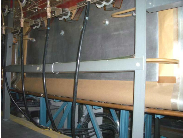
Figure 95. A Shiva bank module after replacement of brown paper below hot bus plate on this half of the module. In addition, a large number of the ¼-in. thick acrylic supports holding up the Mylar sheets on either side of the modules were snapped off, also due to the concussion from the Shiva discharge. Figure 96 shows new supports in place.
