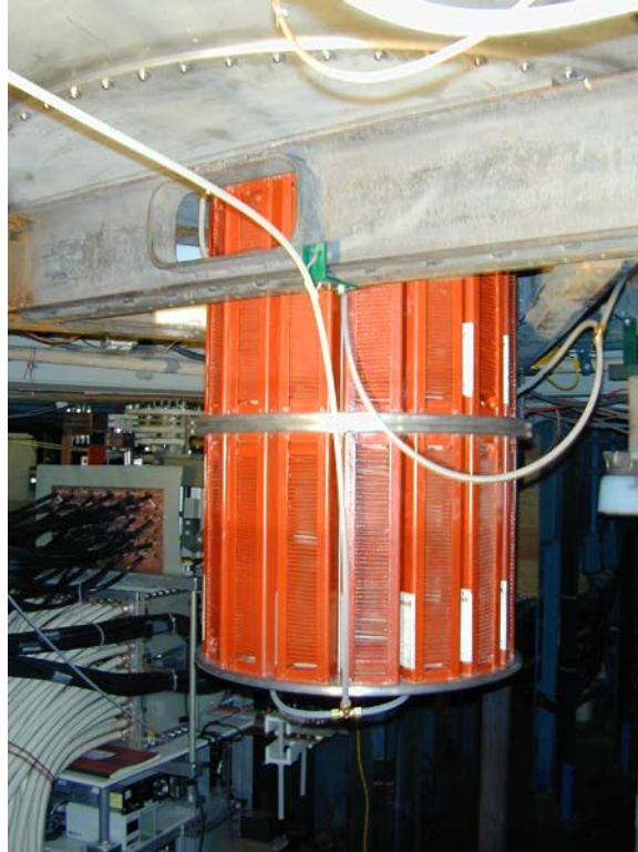
Figure 102. Resistive test load mounted to current-feed plates at center of Shiva bank
