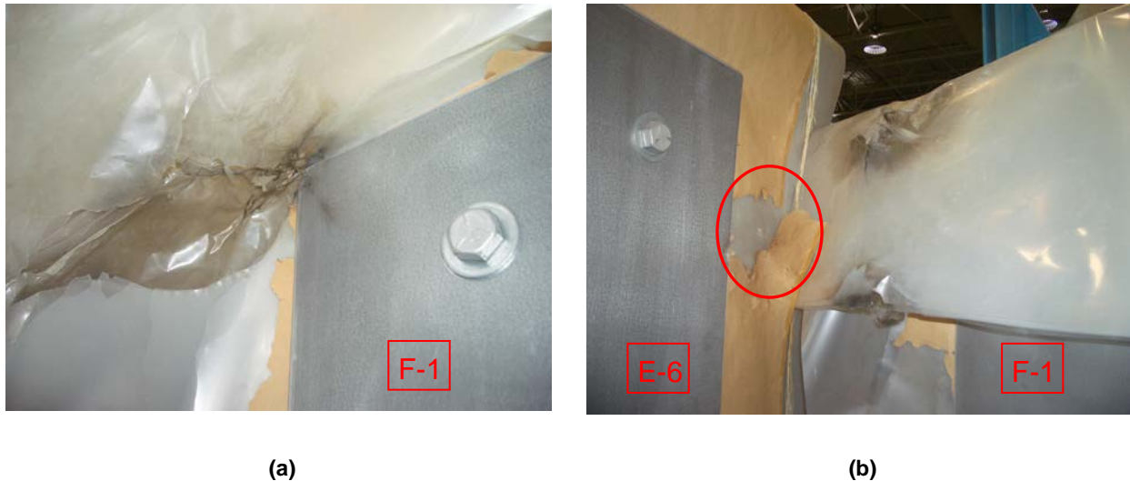
Figure 94. (a) Front and (b) back sides of damaged Mylar on Shiva module F-1
