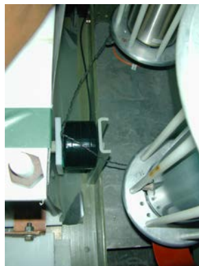
Figure 114. Ignitron-trigger-isolation transformer in place next to Bias bank ignitrons
