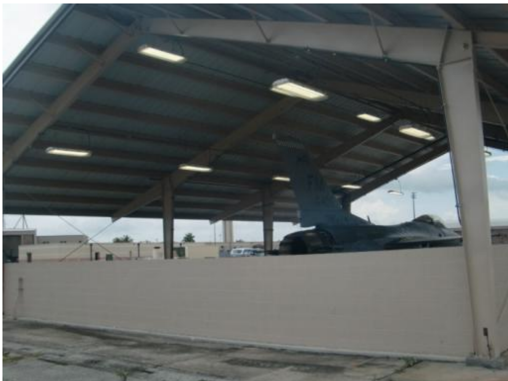
Figure 3. Concrete wall rear of aircraft wash-rack
