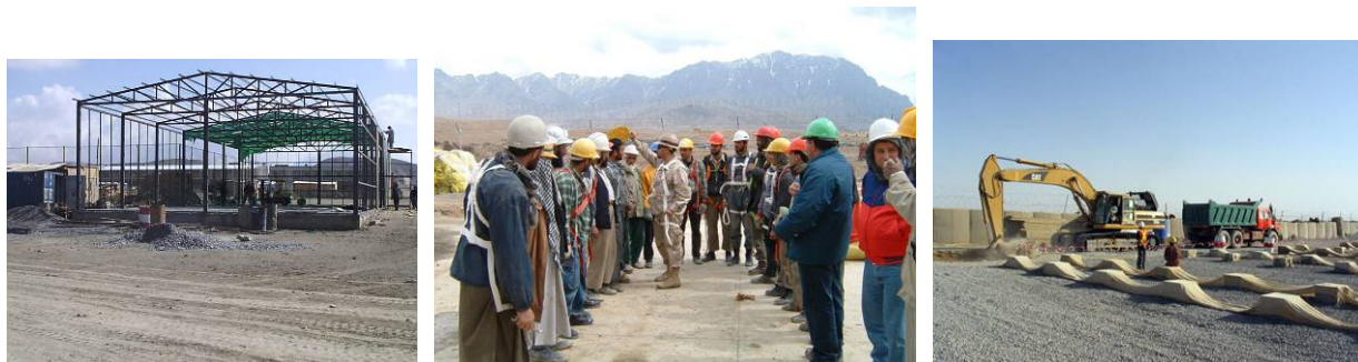
Figure 4. From left: Gym facility being erected at Kabul Military Training Center; Safety training in Pol-e-charki; Digging sewer lines in Kandahar. (Source: USACE – Afghan Engineer District)
