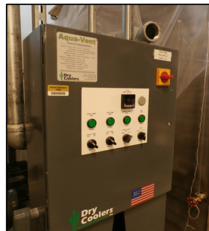
Figure 12. Dry Coolers Cooling System
