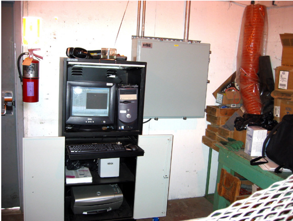
Figure 11. Monitoring control panel and data acquisition computer.
