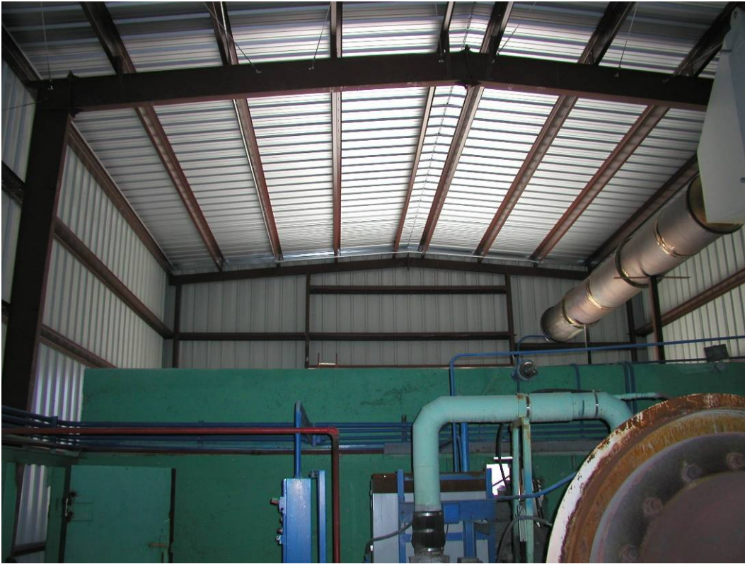
Figure 9. Inside enclosure – discharge end.
