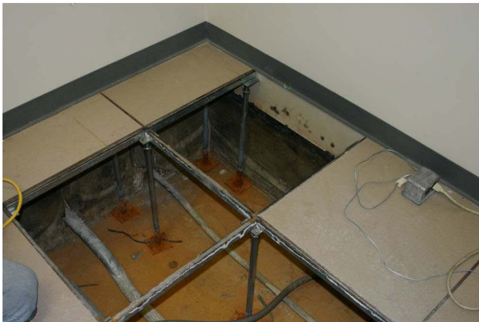
Figure 11. Mold growth on walls under elevated floor.
