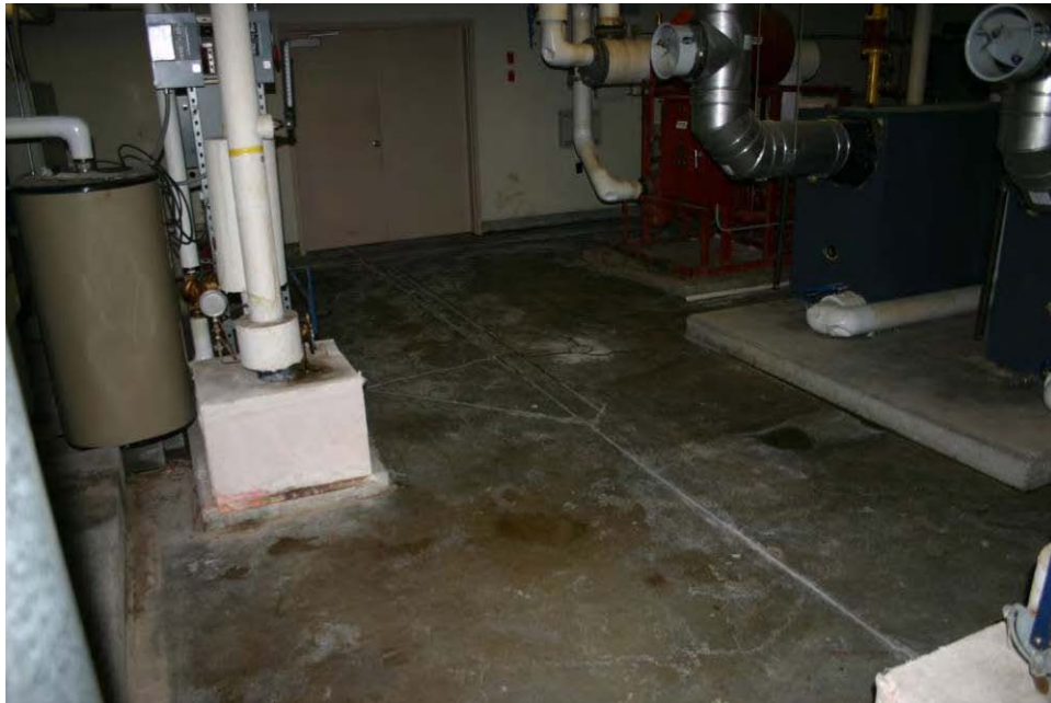
Figure 8. Glycol on floor of Mechanical Room 2.
