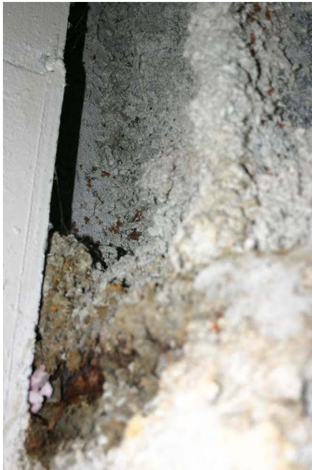
Figure 9. Water on steel column in Mechanical Room 2.
