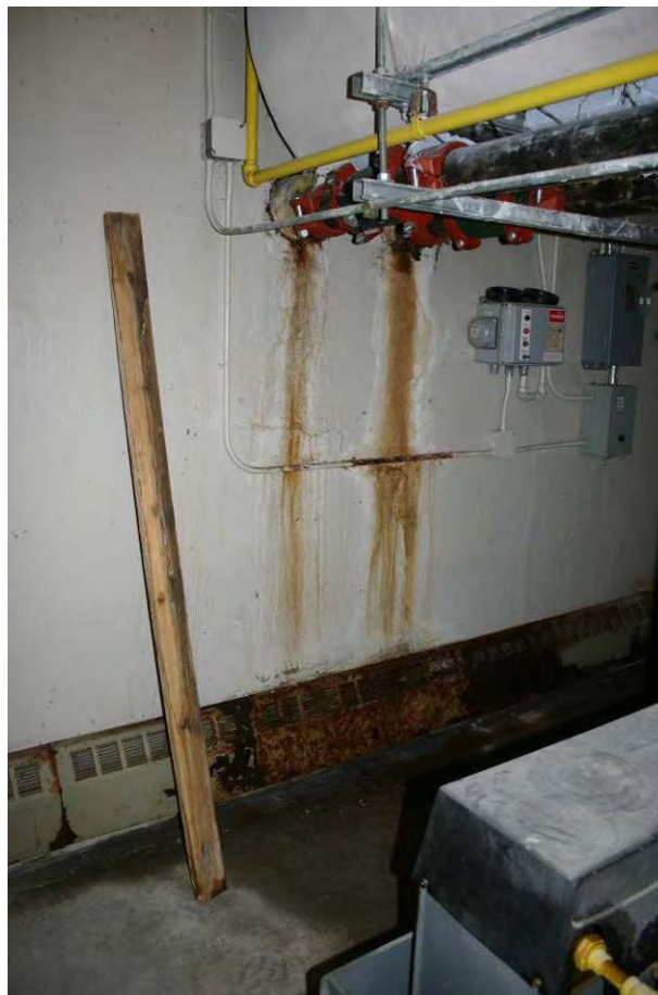
Figure 7. Exhaust and coolant lines through wall in Room B28A.
