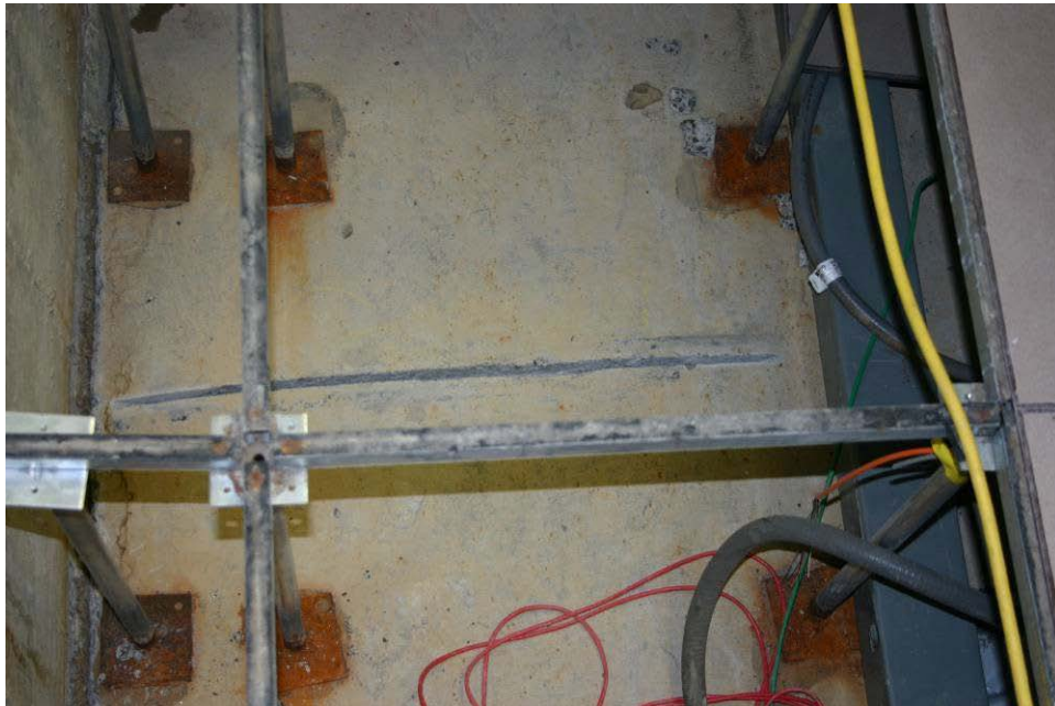
Figure 10. Corrosion of elevated floor supports and frame.
