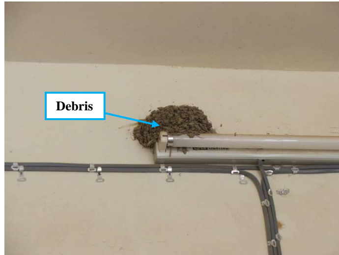
Site Photo 9. Debris on light fixture
