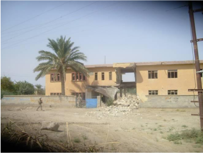
Site Photo 2. Al Iqitadar School destruction (Courtesy MNC-I)
