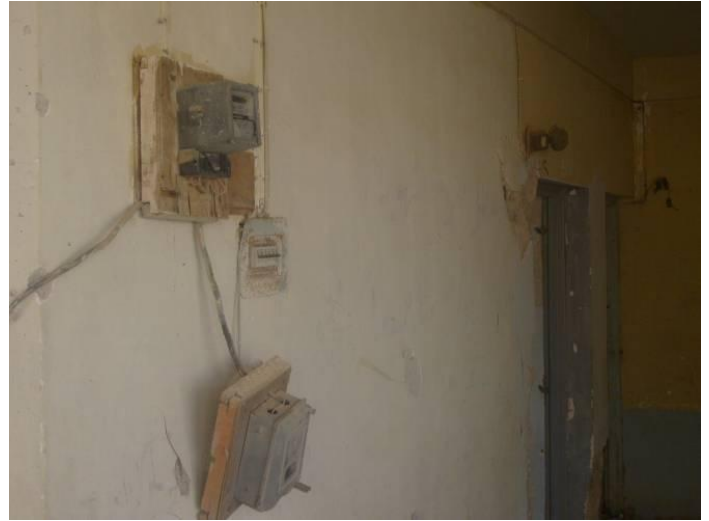
Site Photo 3. Electric panel destruction (Courtesy MNC-I)
