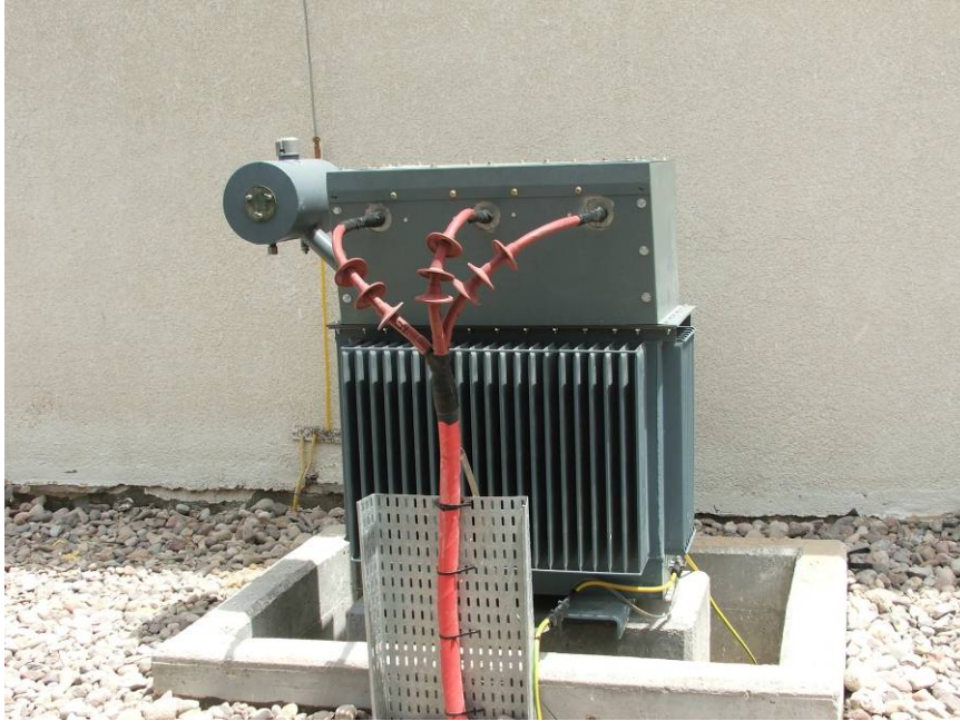
Site Photo 6: 11 to 0.4 kV auxiliary transformers
