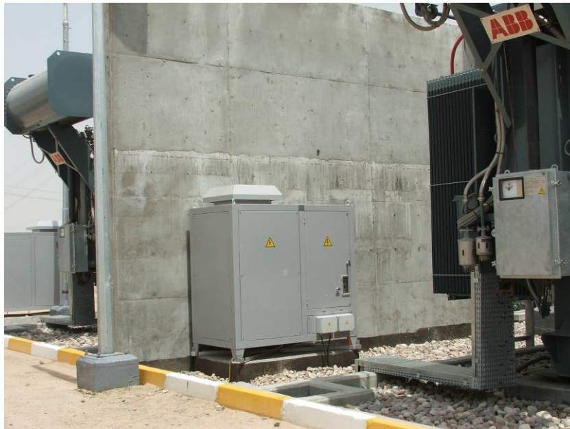
Site Photo 7: Grounding system
