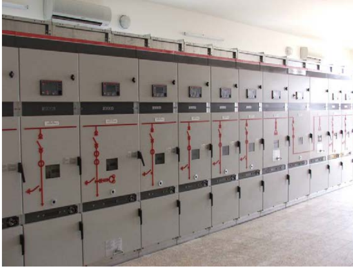
Site Photo 4: 11 kV switchgear
