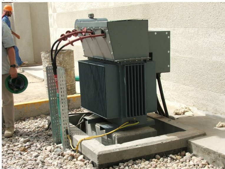
Site Photo 6: 11 to 0.4 kV auxiliary transformers
