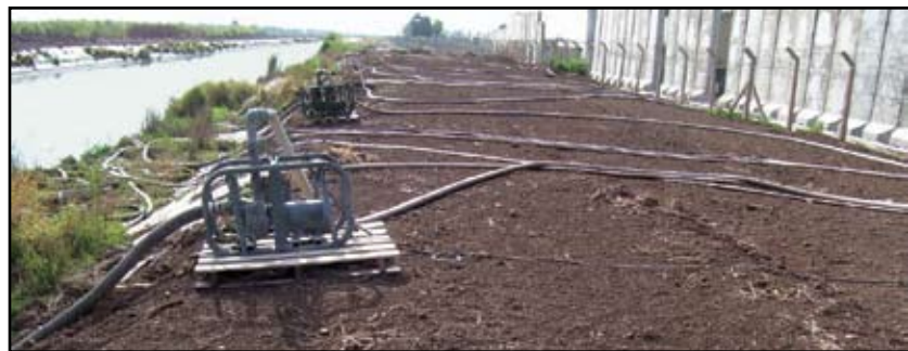
After the engineers laid a solid base of gravel, the 3,000-gallons-per-hour reverse osmosis water purification units (ROWPUs) were placed on skids and protected by concrete barriers.
