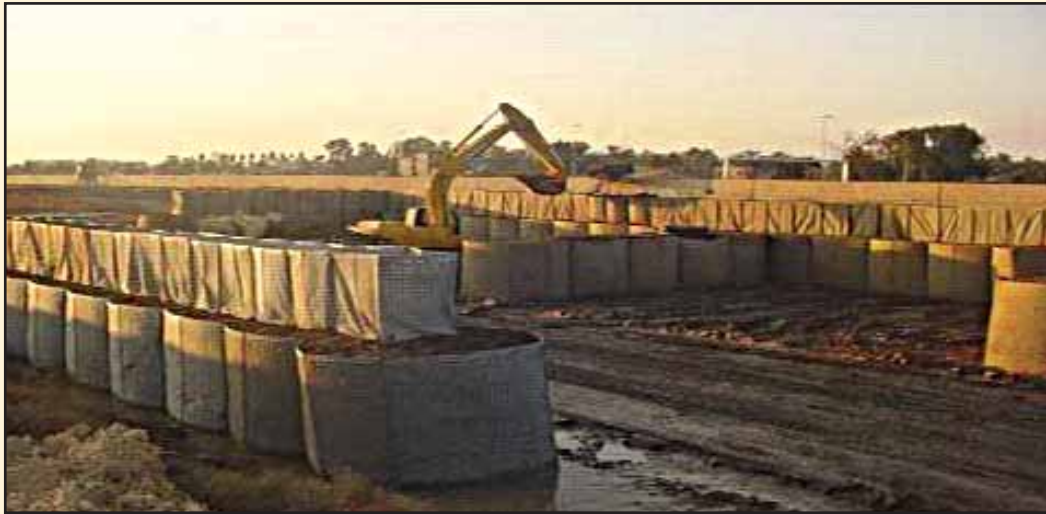
Soldiers of the 63d Ordnance Platoon and A Company, 92d Engineer Battalion, add HESCO barriers to the Liberty ammunition holding site in Baghdad.
