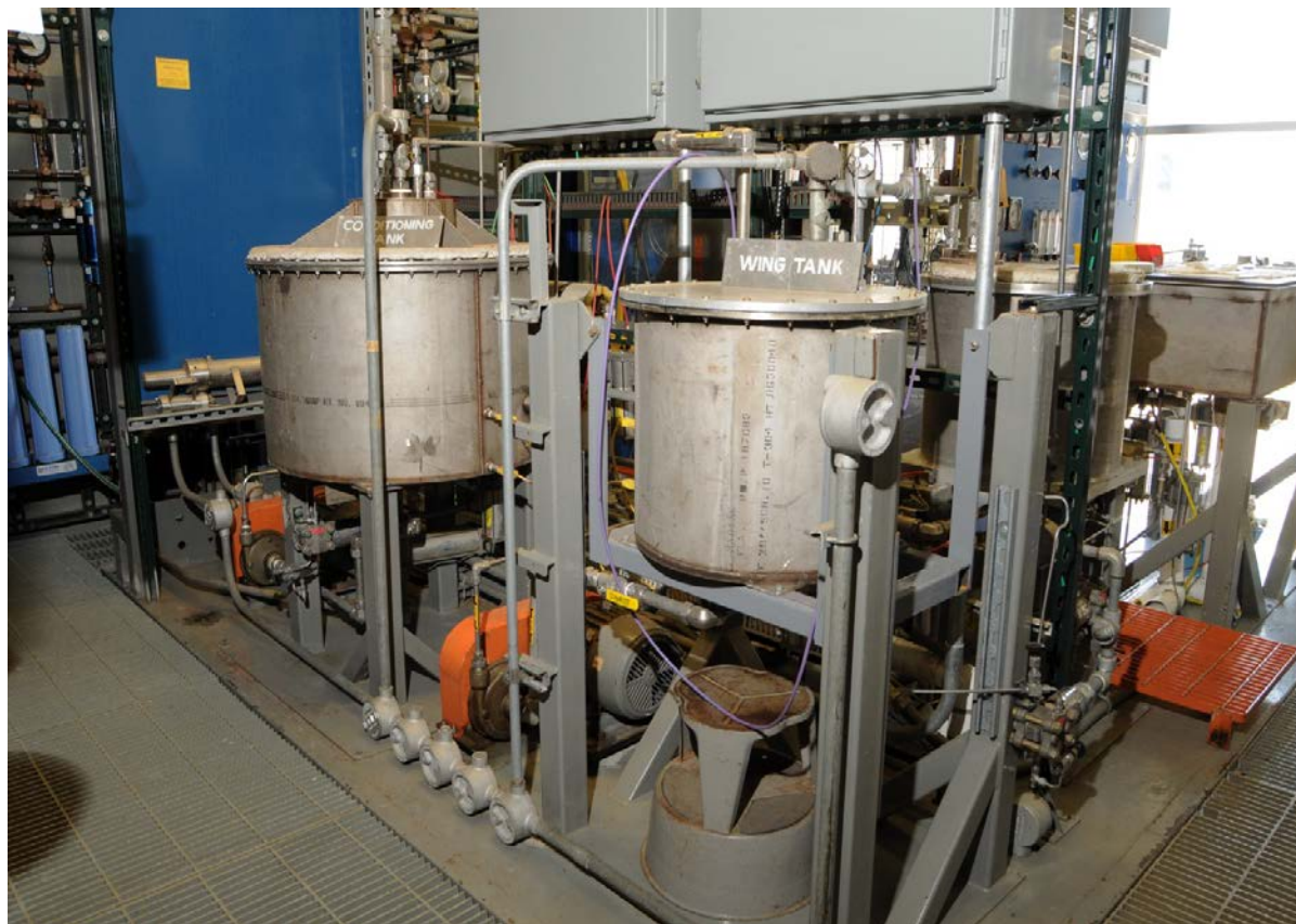
Figure 3 - Conditioning Tank (left) and Wing Tank (right) on the ARSFSS
