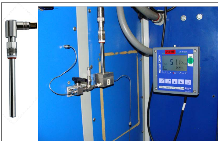
Figure 2 – Dissolved Oxygen Sensor and Placement Location on the ARSFSS Left - Sensor as Uninstalled Right – Sensor as Installed
