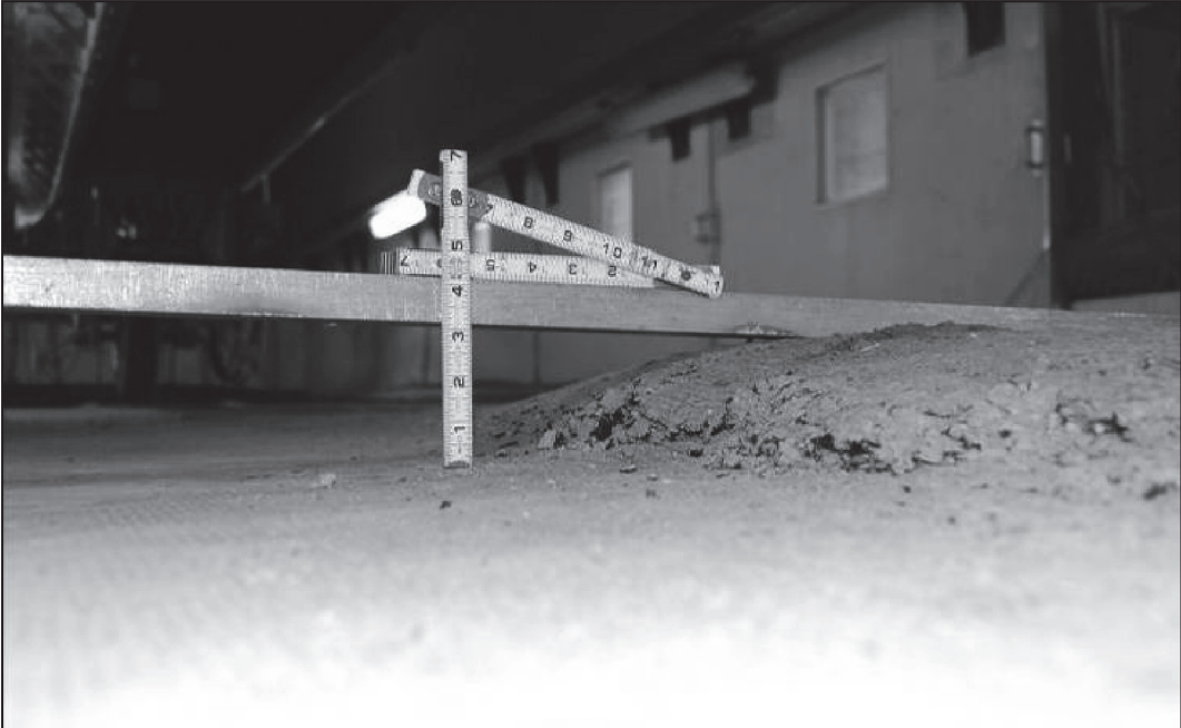
Figure 26. Foamed Asphalt upheaval west side of the rut (@ STA 0+15) after 5,906 passes.
