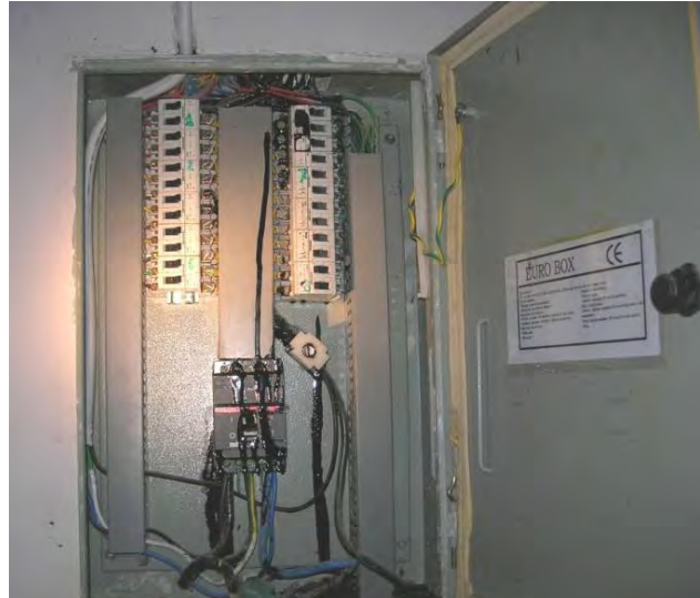
Main Circuit Breaker Panel, LSF-1 (From Army photographs taken on January 2, 2008)
