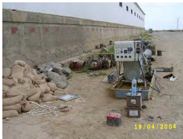
Figure 1. Generator and Housing Area Involved in the Specialist Campo-Siles Electrocution (From Army Photographs)
