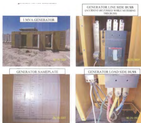
Figure 11. Generator on Which Sergeant Montpetit was Attempting Repair When Electrocuted (From Army Photographs)
