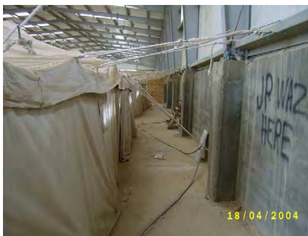
Figure 2. Generator Cable and Housing Unit Involved in Specialist Campo-Siles Electrocution (From Army Photographs)
