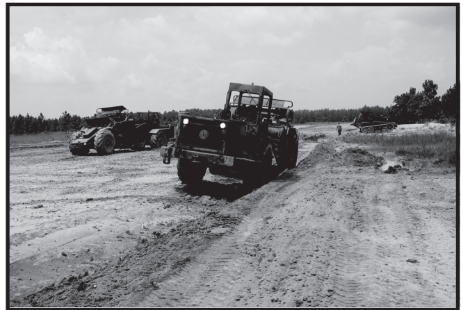
Grading, leveling, and drainage construction operations using the 613BS Scraper and DEUCE
