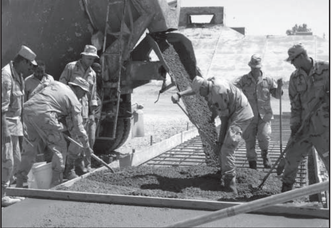
The Minnesota National Guard's 142d Engineer Battalion places concrete for a high-voltage power plant at LSA Anaconda in Balad, Iraq.
