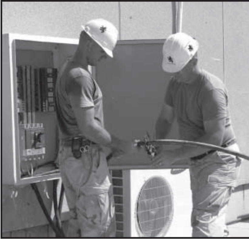
Prime power soldiers from the 249th Engineer Battalion prepare wiring for a branch circuit to refrigerate Army and Air Force Exchange Service storage containers.
