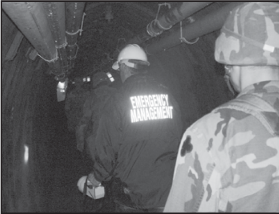
Soldiers and members of the Office of Emergency Management conduct a joint tunnel inspection.
