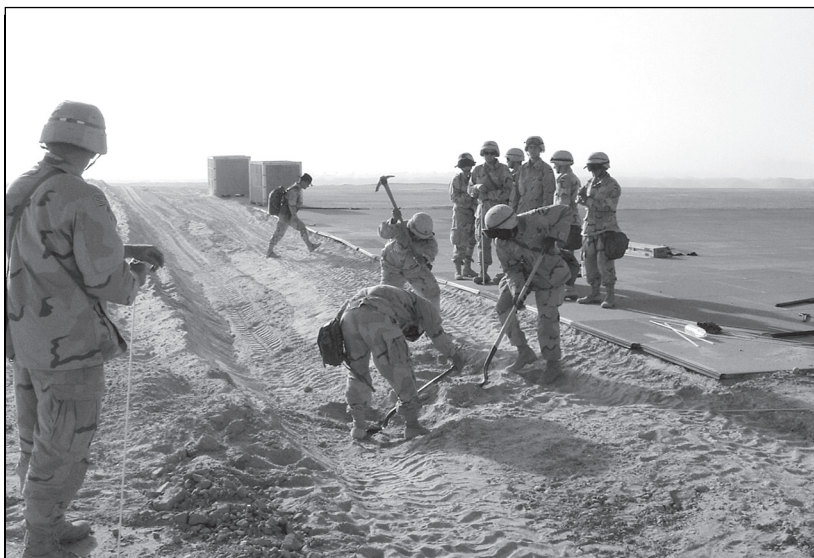
Soldiers from a pipeline company repair matting that buckled in the extreme desert heat.
