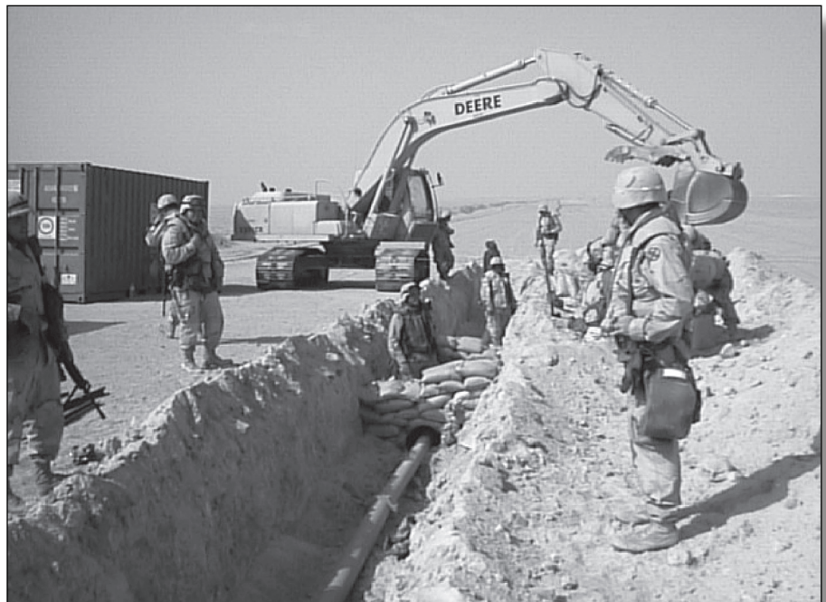
At crossing sites, the pipeline is buried deep enough that the weight of passing vehicles won't affect it.
