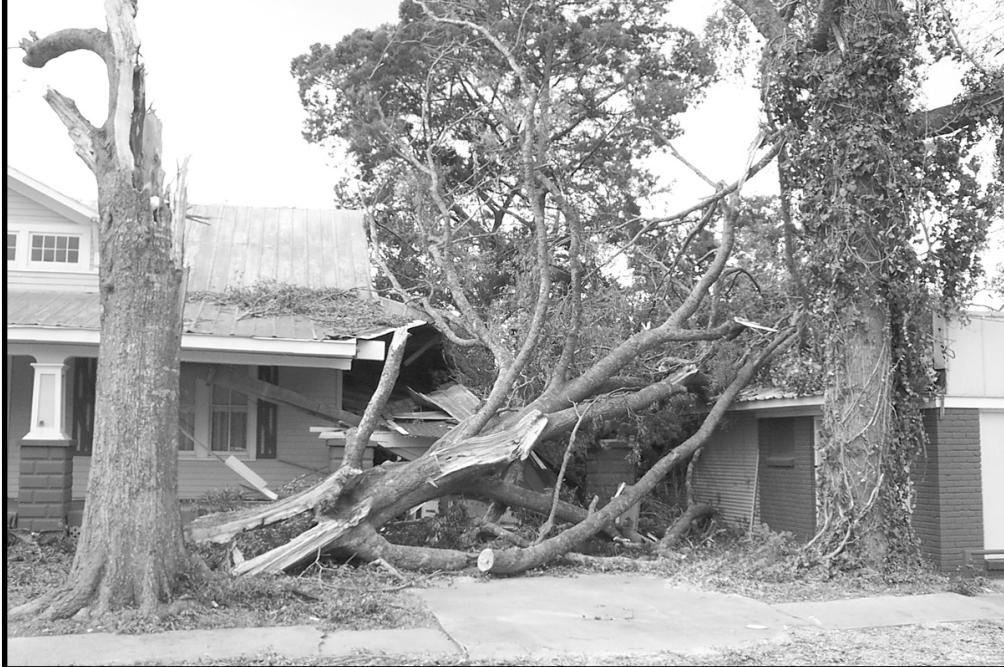
Hurricane Lili caused widespread damage to civilian housing in October 2002.
