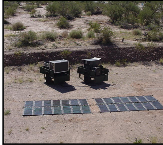
Figure 6 Thin Film Solar Panels with Field Generators
