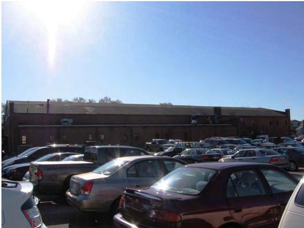
Photo 2: West Façade with Deteriorating Roof
