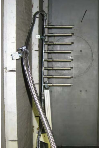
Figure 2.16: CO 2 distribution manifold installed in the TGF [12]
