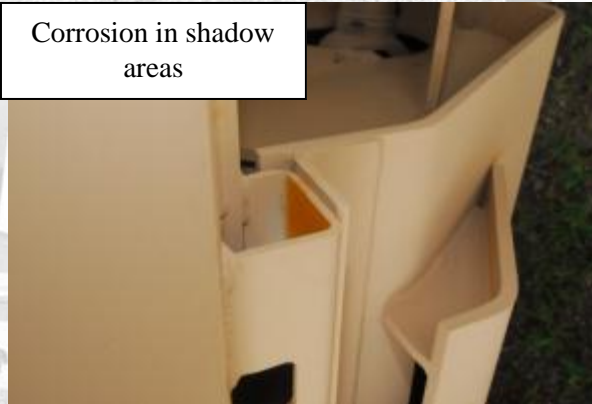
Corrosion in holes and recesses
