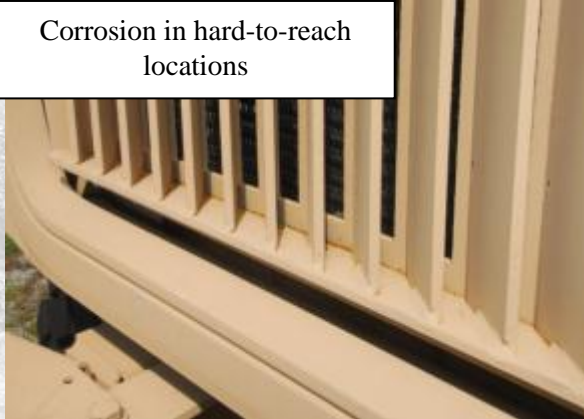
Corrosion and particles in V Hull drain
