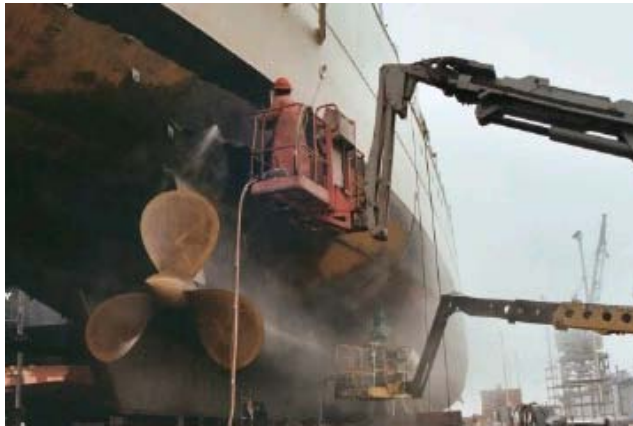
High Pressure Water Jet
