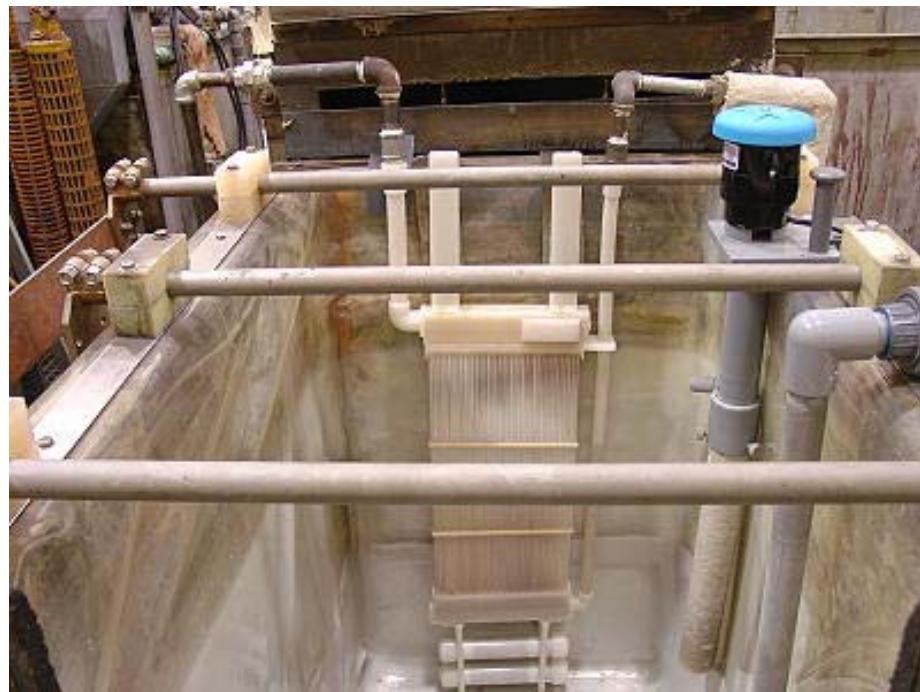
290 gal Dem/Val plating tank
