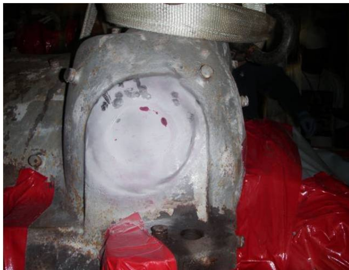
FIGURE 2: CIRCUMFERENTIAL CRACKING IN PLUG
