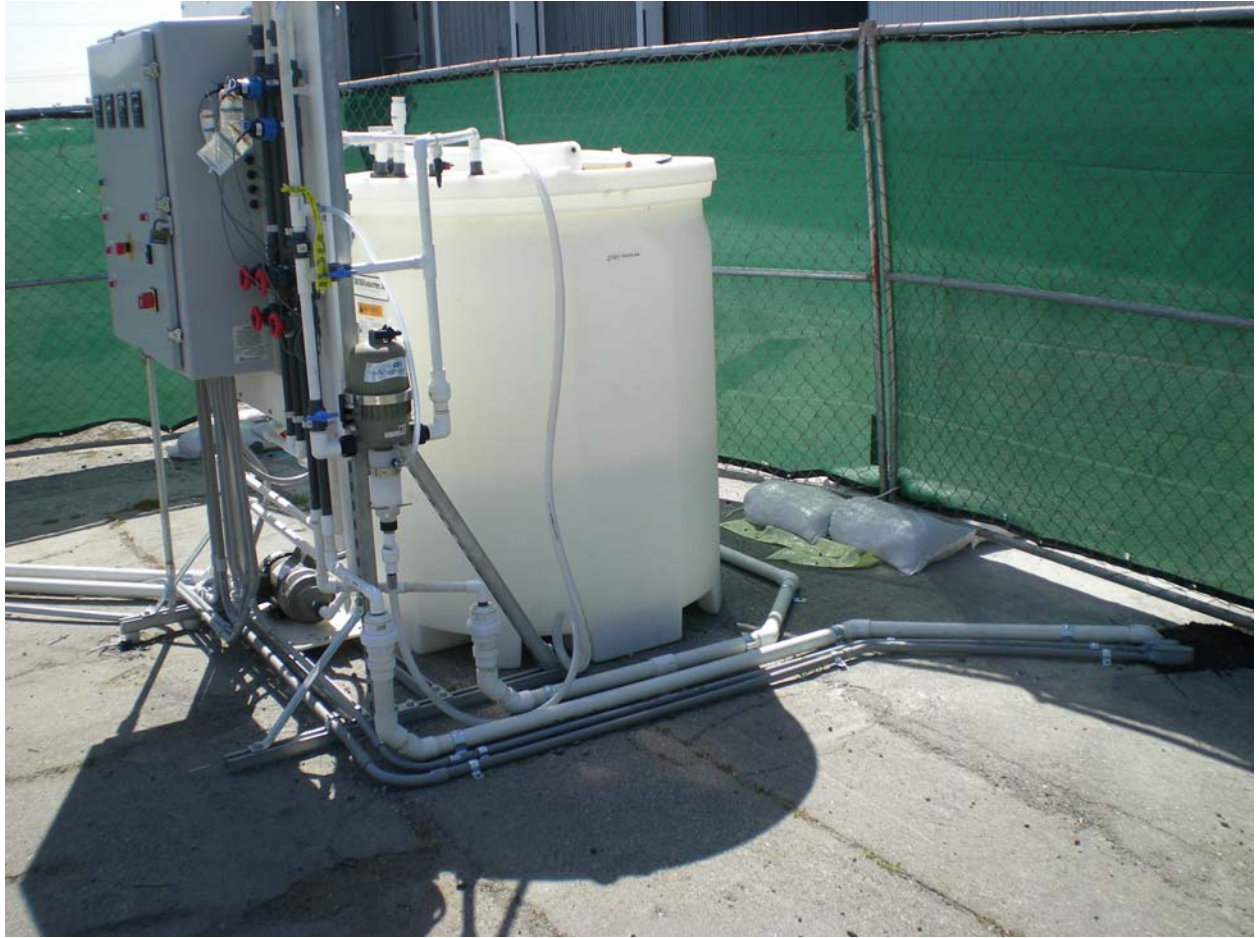
Picture 20. Surge tank and control panel side.
