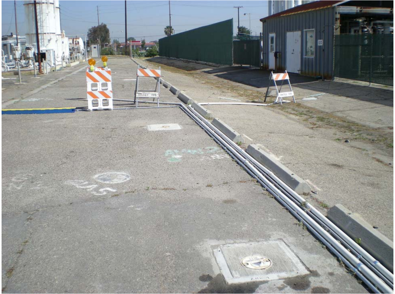
Picture 14. Piping between injection and extraction wells.
