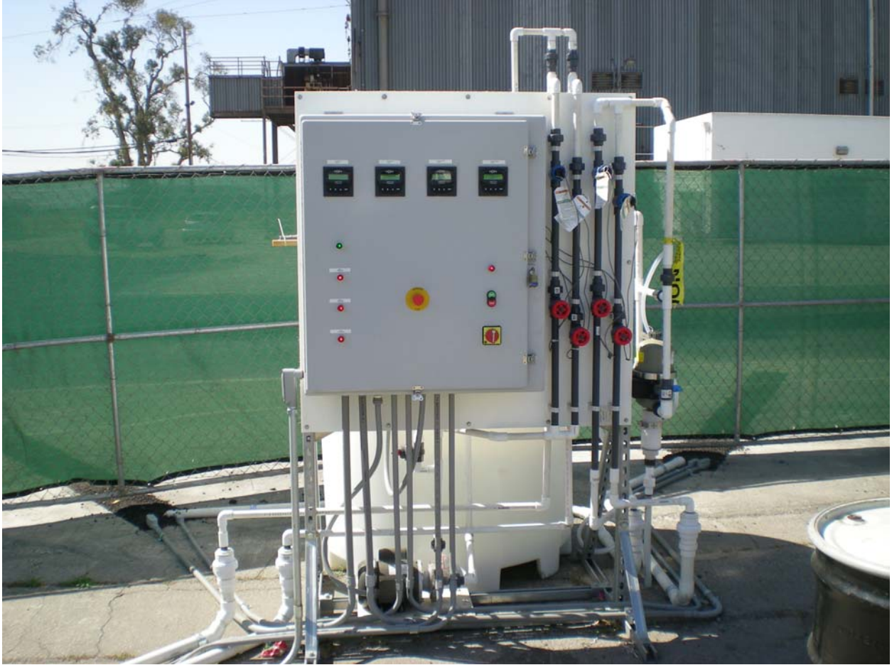
Picture 18. Surge tank and control panel front.
