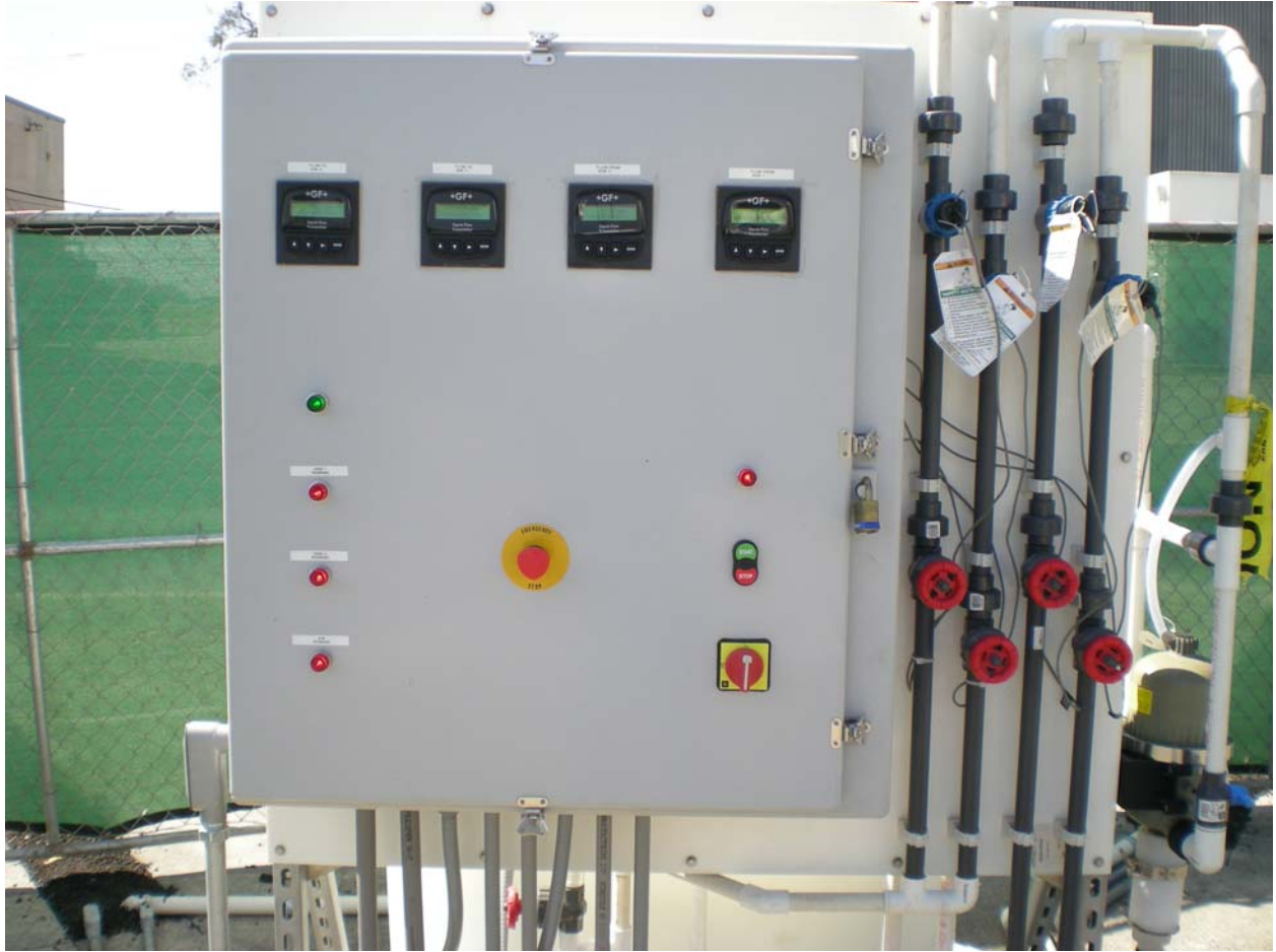
Picture 3. Injection system control panel.
