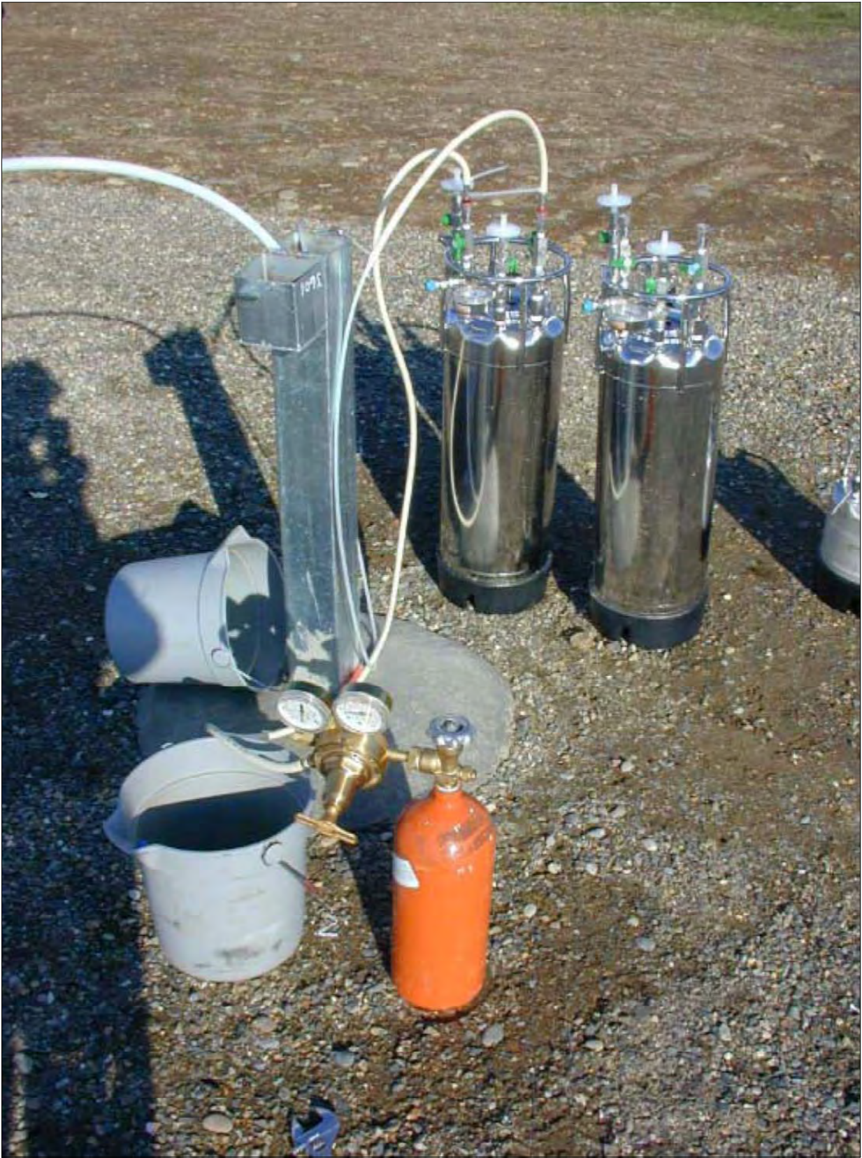
Figure 5-4 BACTERIA INJECTION SYSTEM EXAMPLE ER-0513 FINAL REPORT SEAL BEACH NAVAL WEAPONS STATION, SEAL BEACH, CA
