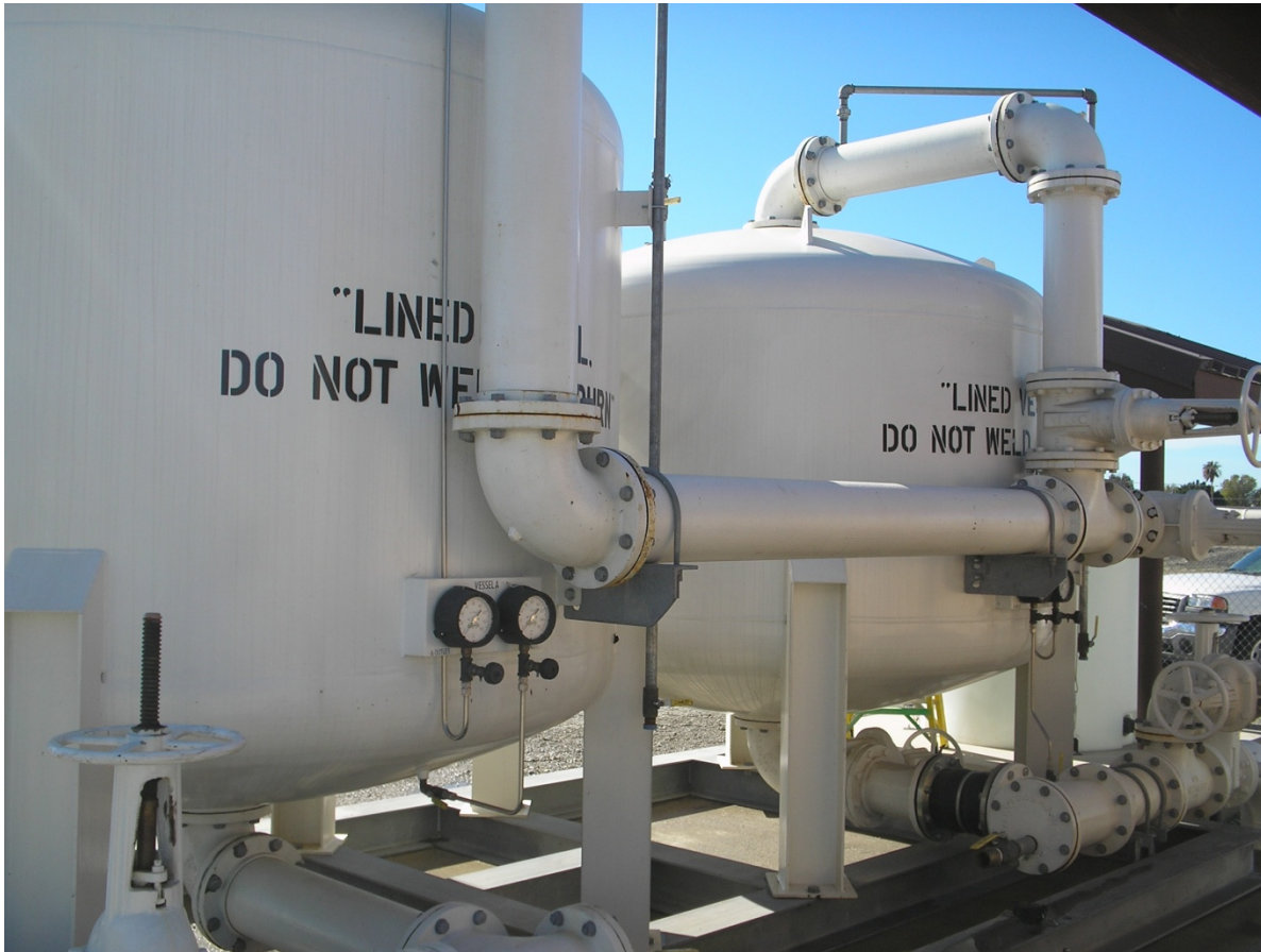
Figure 12. Face piping and well connection – WVWD.
